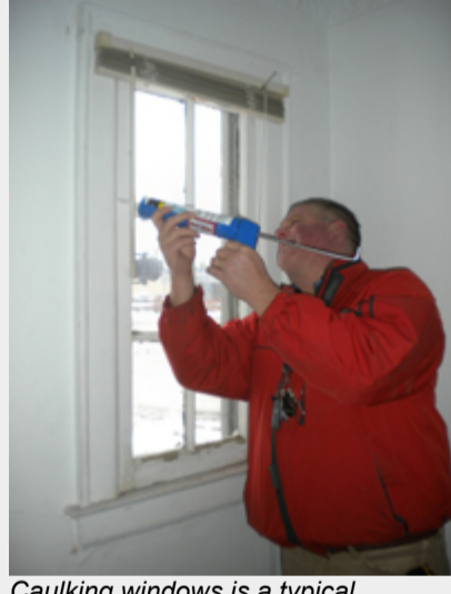
Caulking windows is a typical weatherization service that helps lower energy bills.
